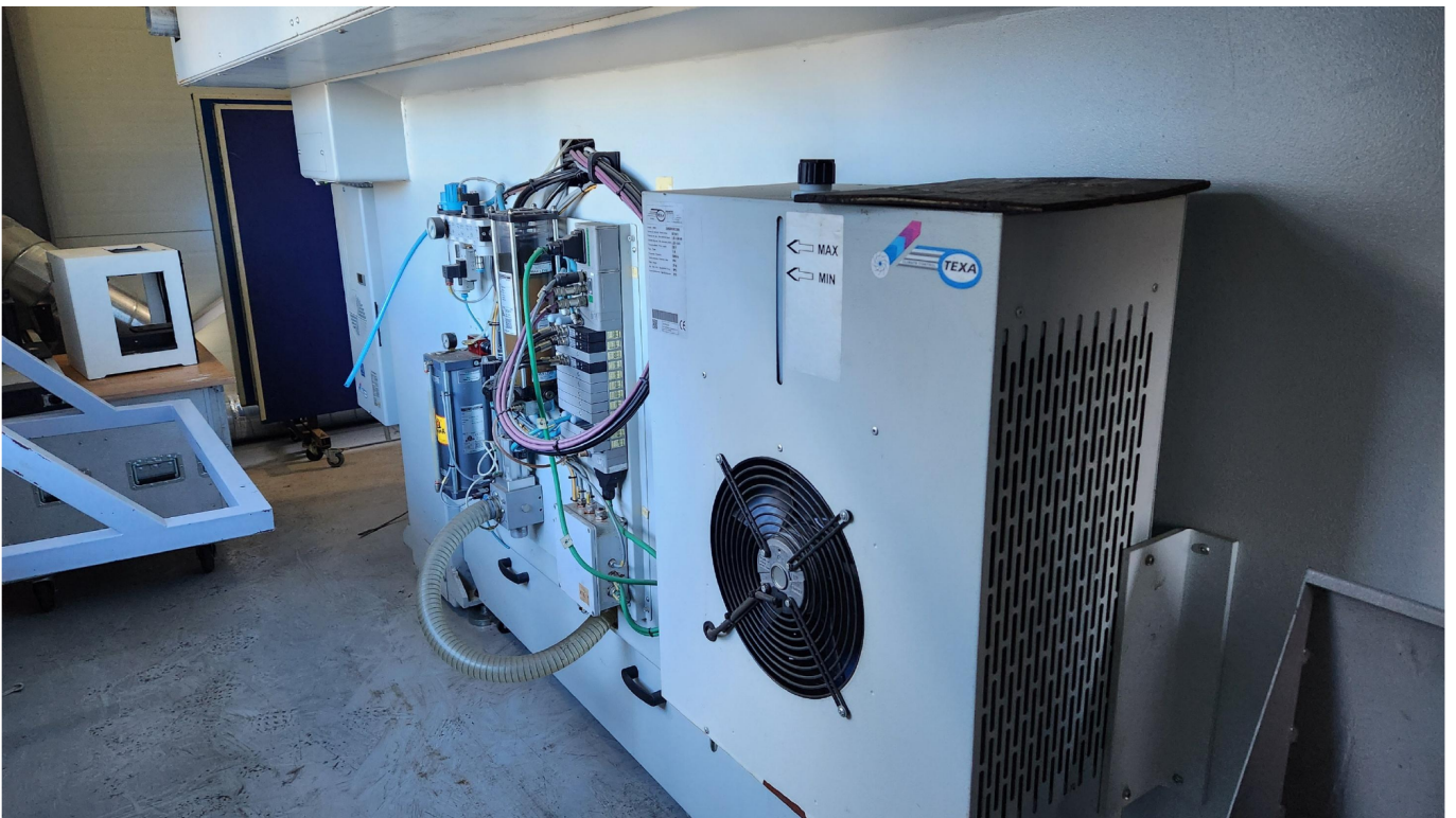
Equipment Detail - View 7
