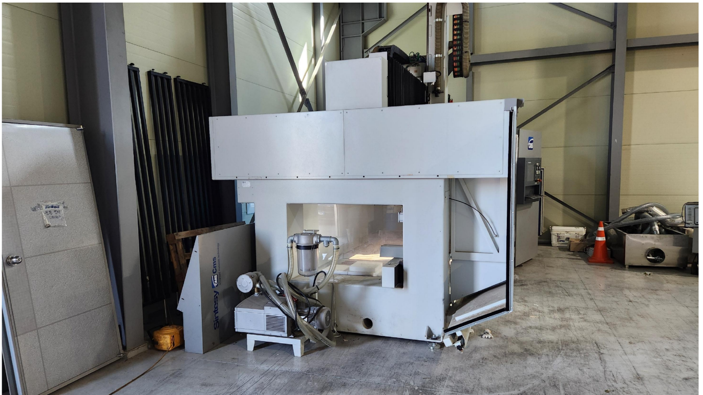
Equipment Detail - View 8
